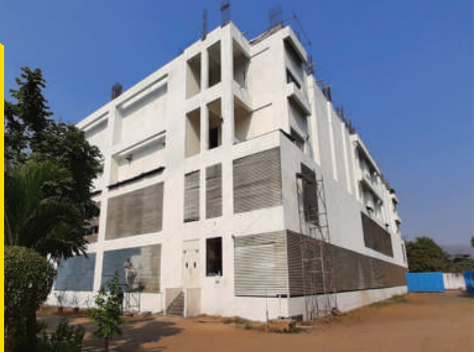
MUMBAI DATA CENTER
