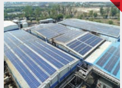
Rooftop Solar, MIL Hapur
