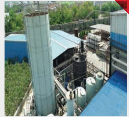
RO plant for water filtration and recycling in Hapur
