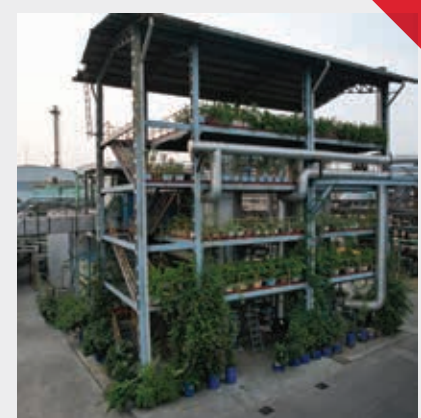
Hot Water generation system of Co-Gen Plant, Hapur
