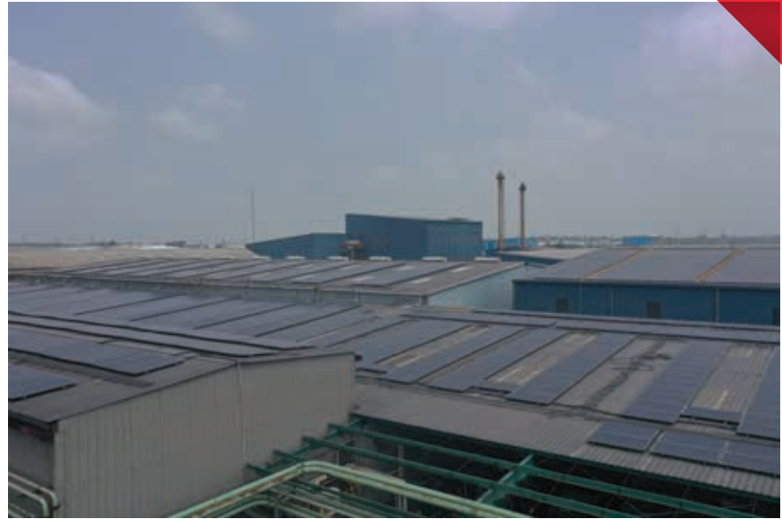
Rooftop Solar System MIL Rohad (H.R.)
