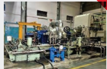
Biomass based Turbine, Hapur
